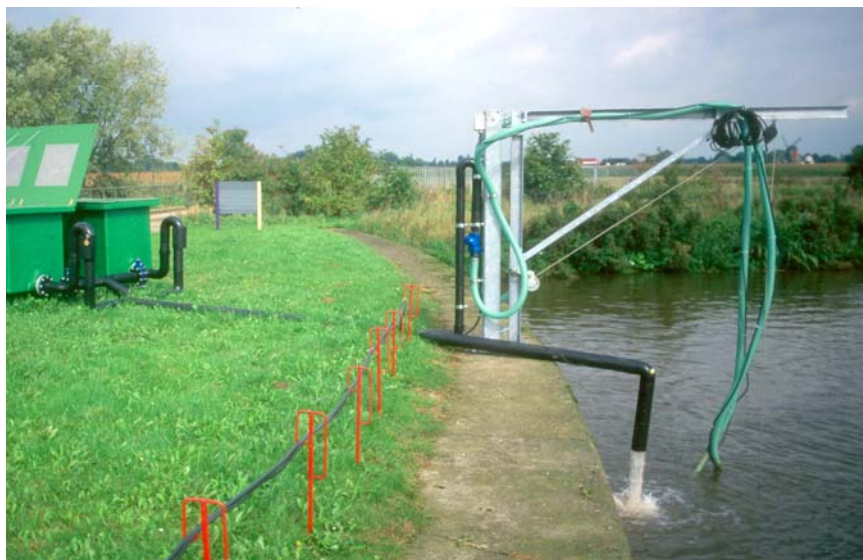
Figure 10 Pumps and outlet of the Migromat® at Alphen hydropower station.
