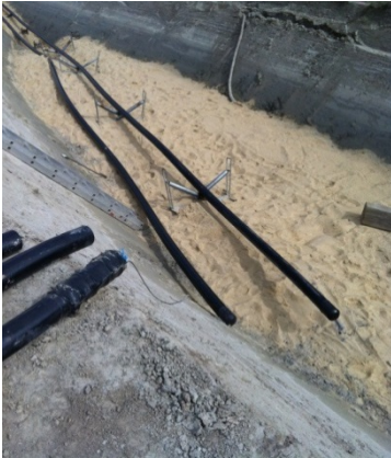
Figure 20 Cable ends in jointing pit
